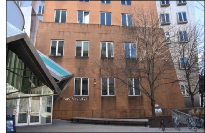
TYPICAL BRICK MASONRY STAINING
