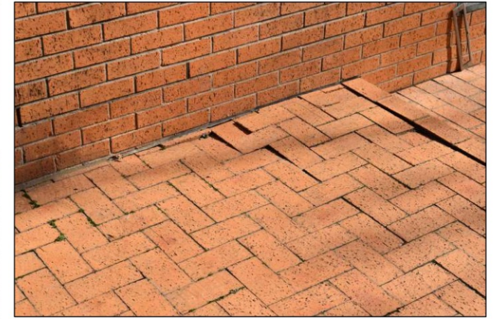
TYPICAL DISPLACED PAVERS
