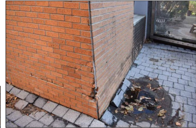
IMPACT DAMAGE AT SOUTHWEST CORNER OF DREYFOOS SOUTH TOWER
