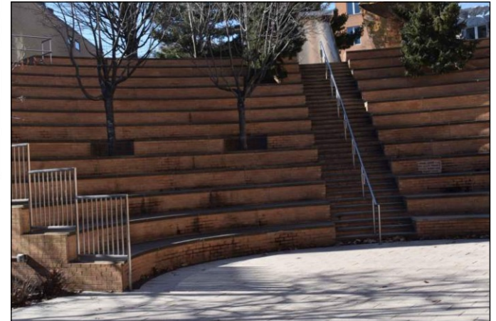
TYPICAL BRICK MASONRY DISCOLORATION AT AMPHITHEATER
