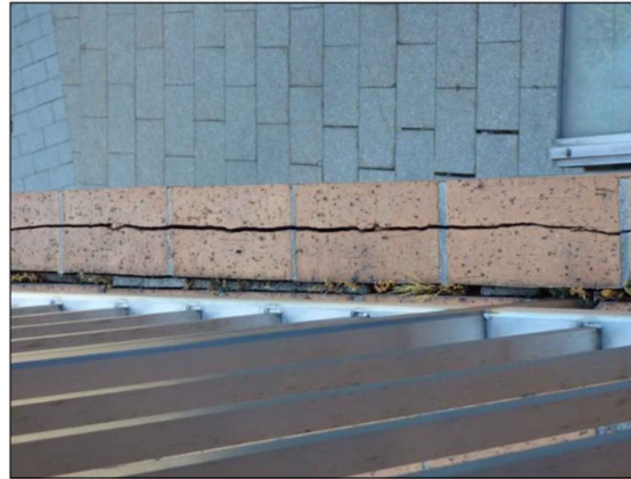
CRACK THROUGH BRICK MASONRY AT EAST ENTRY
