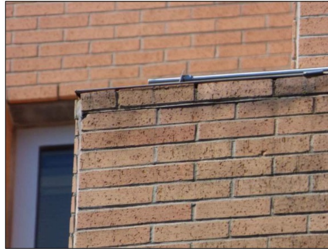
DETERIORATED MORTAR AND DISPLACED TOP COURSE OF MASONRY
